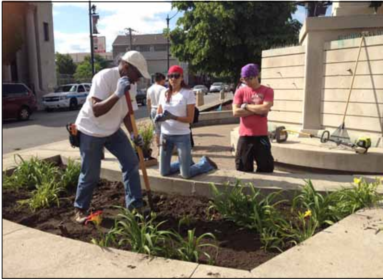
Residents of Pilsen gathered around the Plaza Tenochtitlan Wednesday morning to begin work on the renovation that will offer ample green space and pedestrian accessibility.
