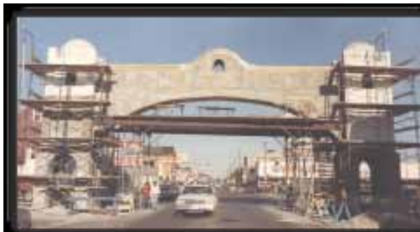
Mexican Arch surrounded by scaffolding and planks near its final rough stages of completion.
